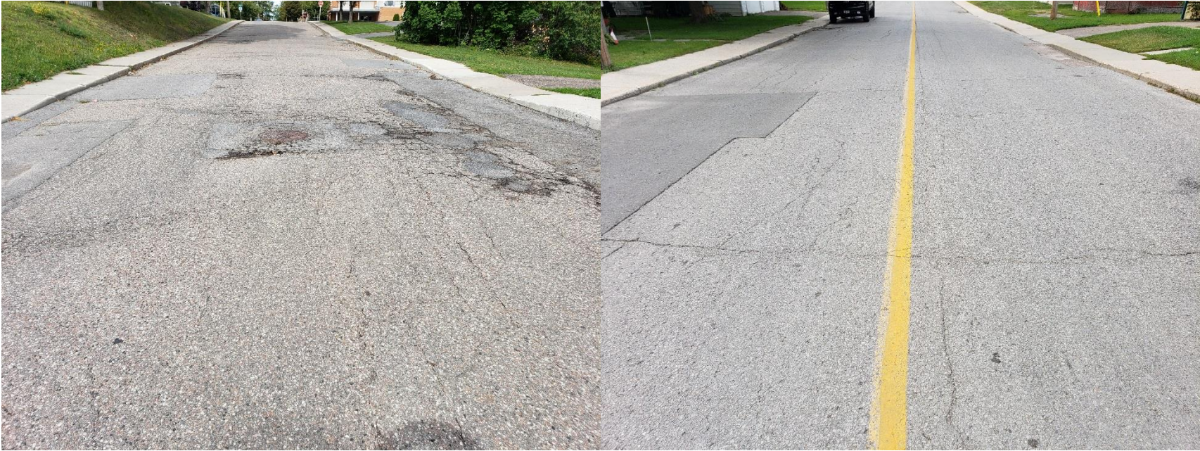
Sample Serious/Failed Road (0-25) (Grey & Dark Red)
